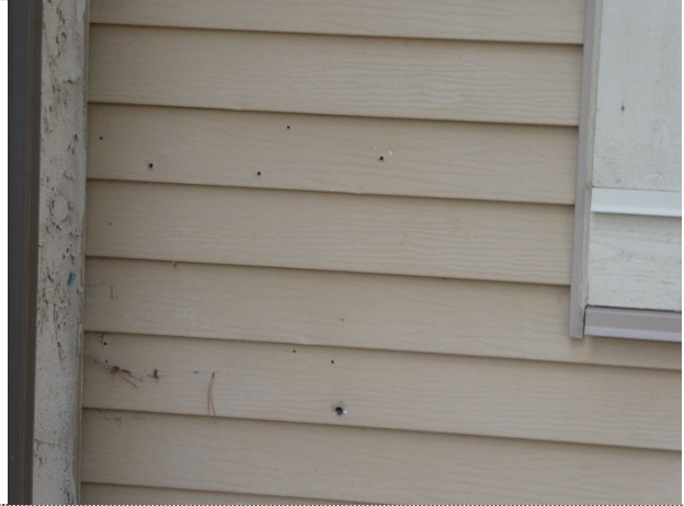
Holes in metal siding
