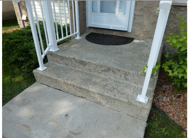
Front entrance step evidencing deterioration
