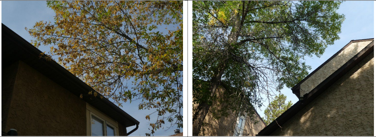
Trees scraping against building components
