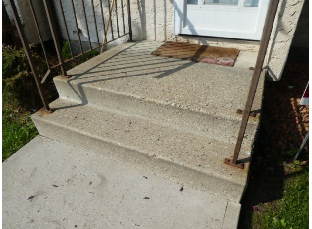
Front step spalled
