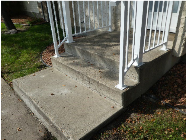
Front entrance step evidencing spalling
