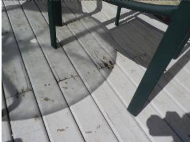
5 Significant deterioration at joints & screw penetrations
