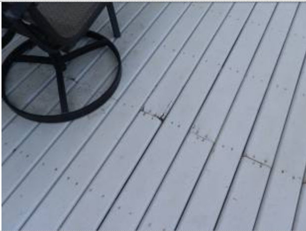
12 Deterioration at joints where screws penetrate
