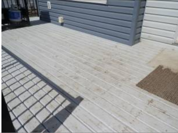
1 Minor deterioration at joints
