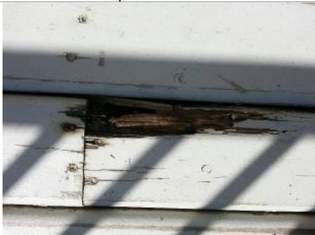
7 Deterioration of wood
