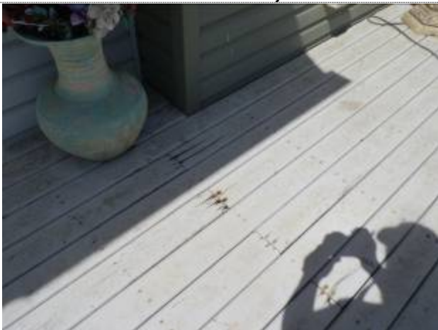
23 Deterioration at joints where screws penetrate
