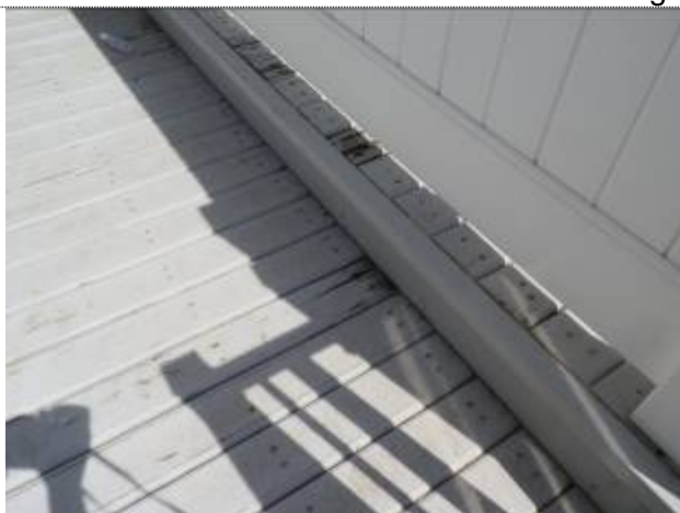
9 & 11 Deterioration at end of deck boards at screw penetrations
