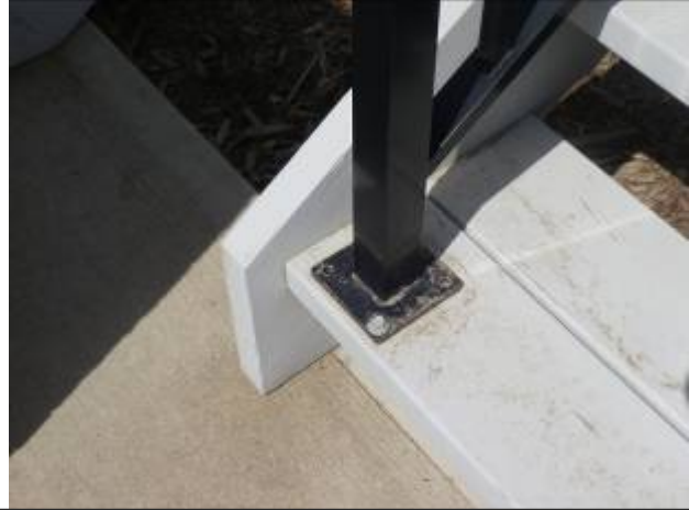
3 Missing bolts in railing
