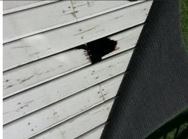
7 Significant deterioration and rot of deck boards
