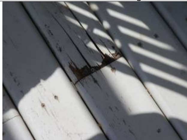
25 Deterioration at joints where screws penetrate
