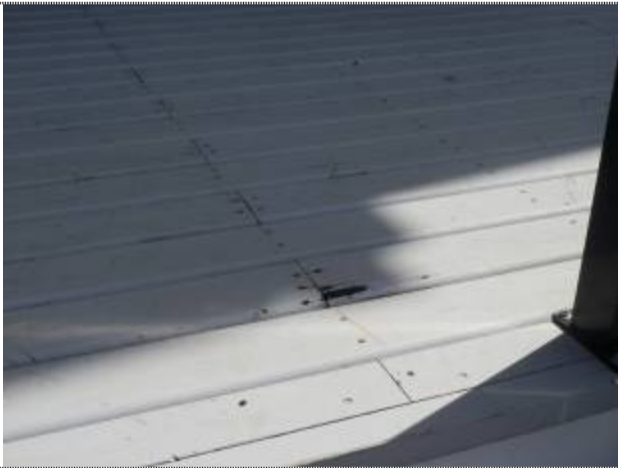
20 Deterioration at joint
