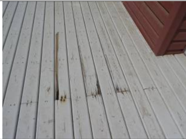
17 Deterioration at joints where screws penetrate Gouge in decking
