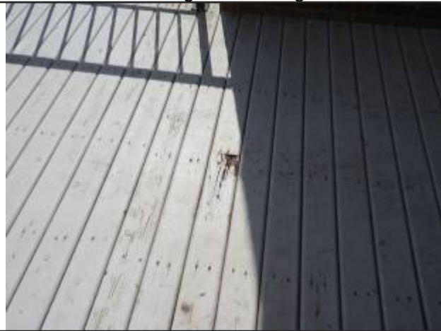
21 Deterioration in decking
