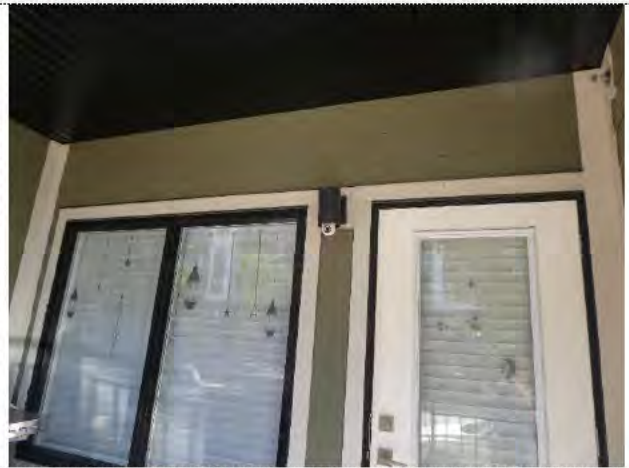
Exterior unit lighting
