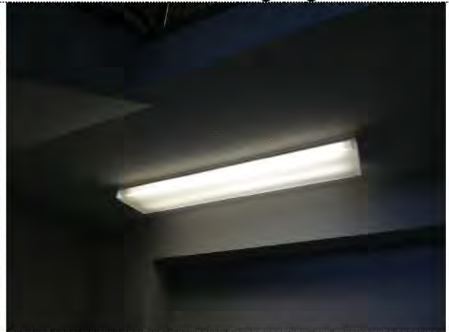
Interior fluorescent lighting
