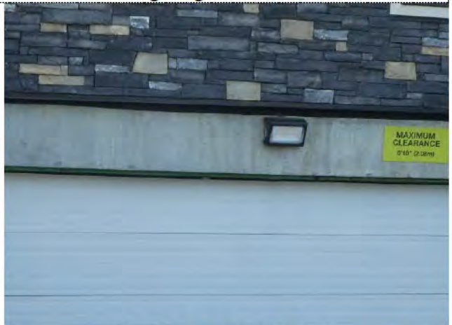
Exterior building lighting
