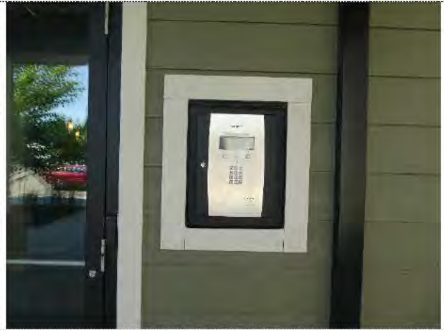
Back intercom panel
