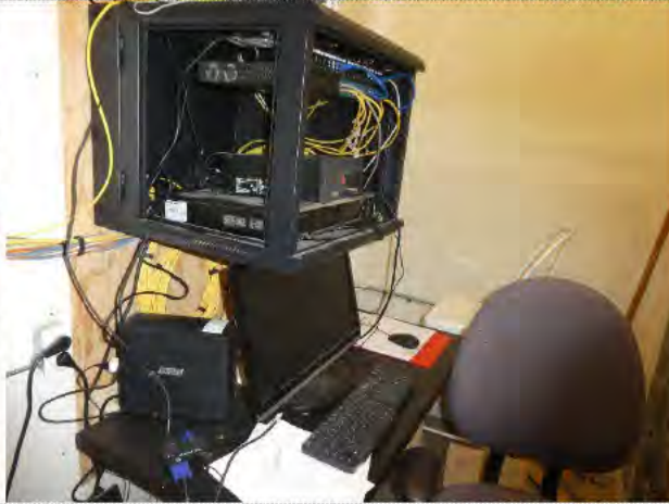
Security camera system
