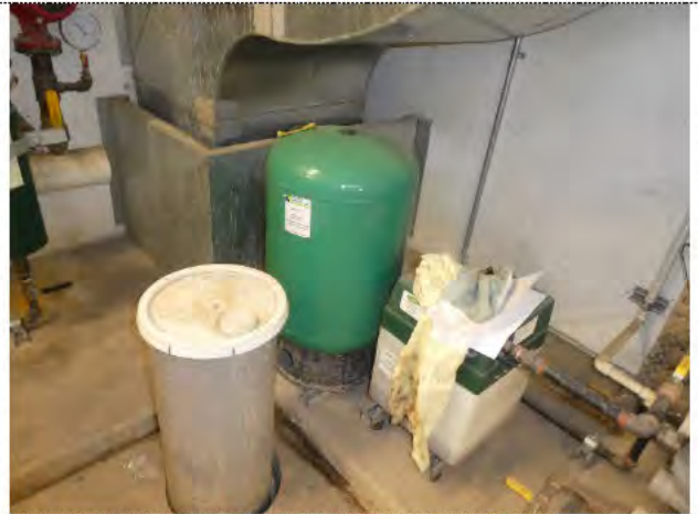
Expansion tank & system feeder
