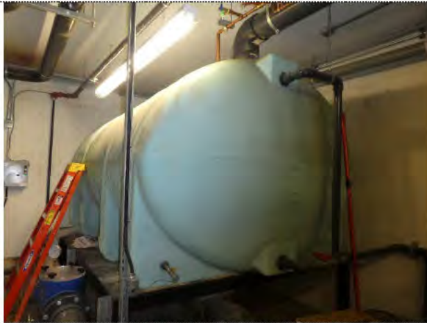
Water holding tank
