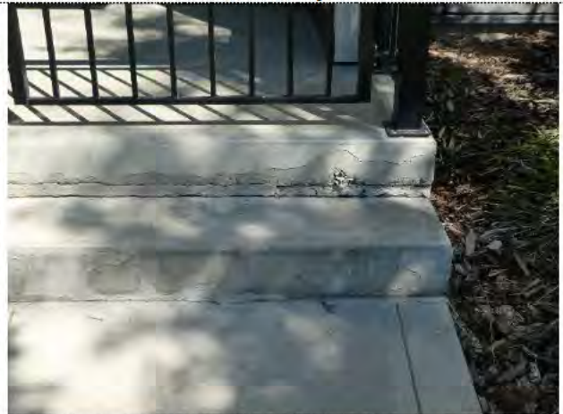
Deteriorated finish on patio steps
