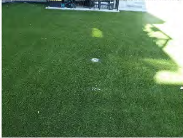
Drain in landscaping (above parkade membrane)
