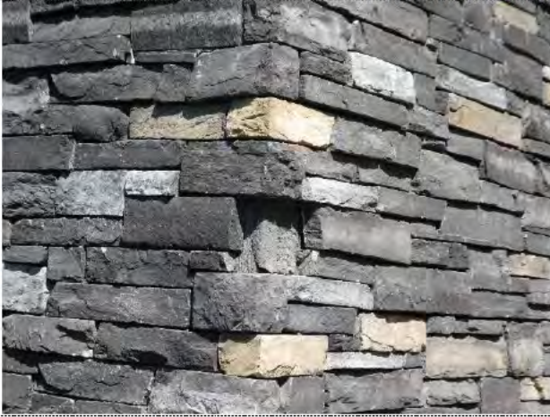
Missing stone veneer
