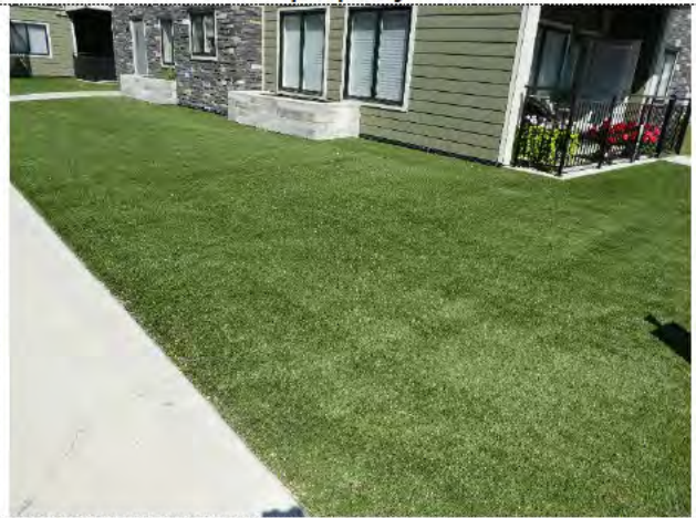
Parkade membrane below artificial grass in courtyard
