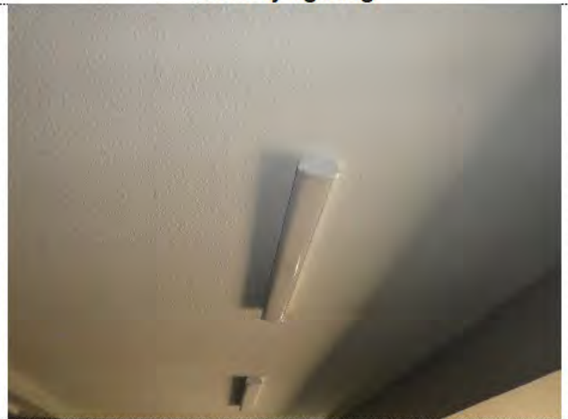
Interior lighting in amenities room
