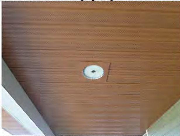
Exterior building lighting
