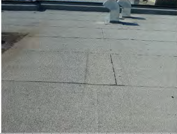
Ridging evident in roofing
