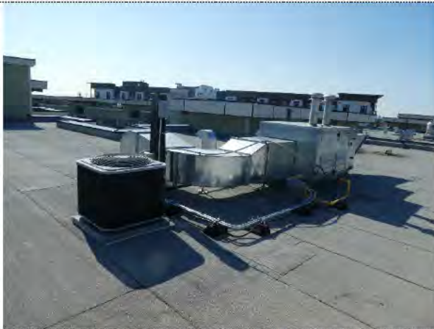
CaptiveAire Indirect Industrial Heater (makeup air unit) & KeepRite A/C unit
