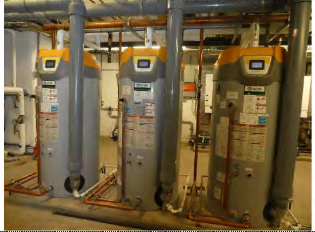
A.O.Smith hot water heaters – 119 Gal M: BTH-400A 300 S: 1741107849623, 1732107107451 & 1741107849621
